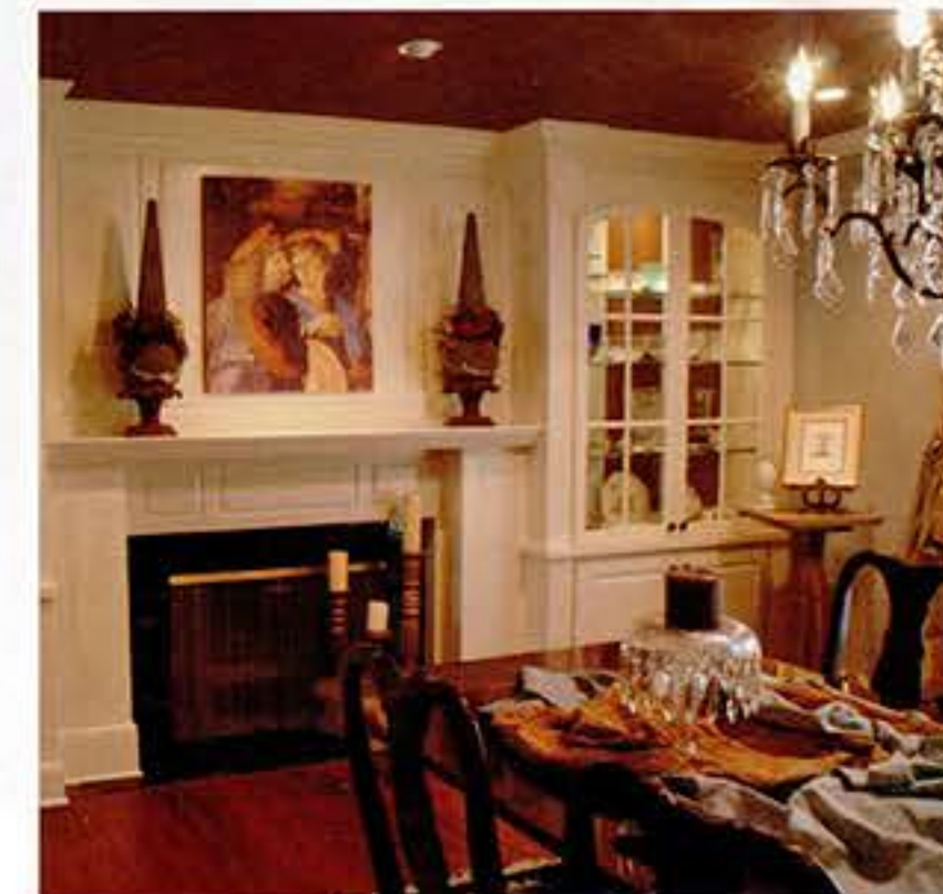
Crews constructed custom built-ins to match those already in what was the home's living room, but now serves as a formal dining area.
